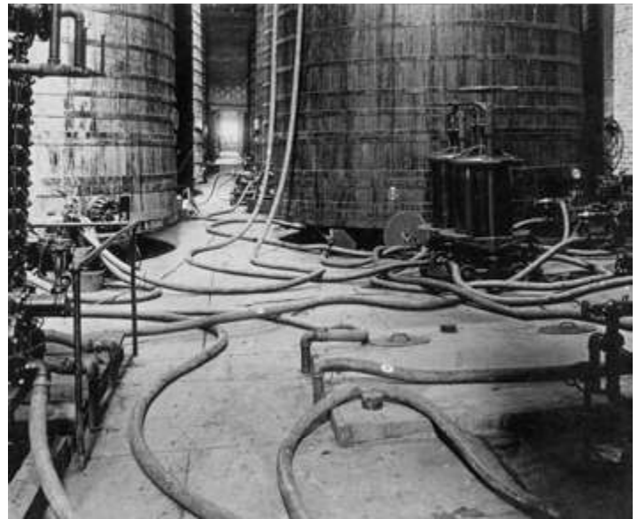
An interior shot of a Lachman & Jacobi Winery storage building in Petaluma shows the network of hoses, large tanks, and piping used for wine storage and blending.
